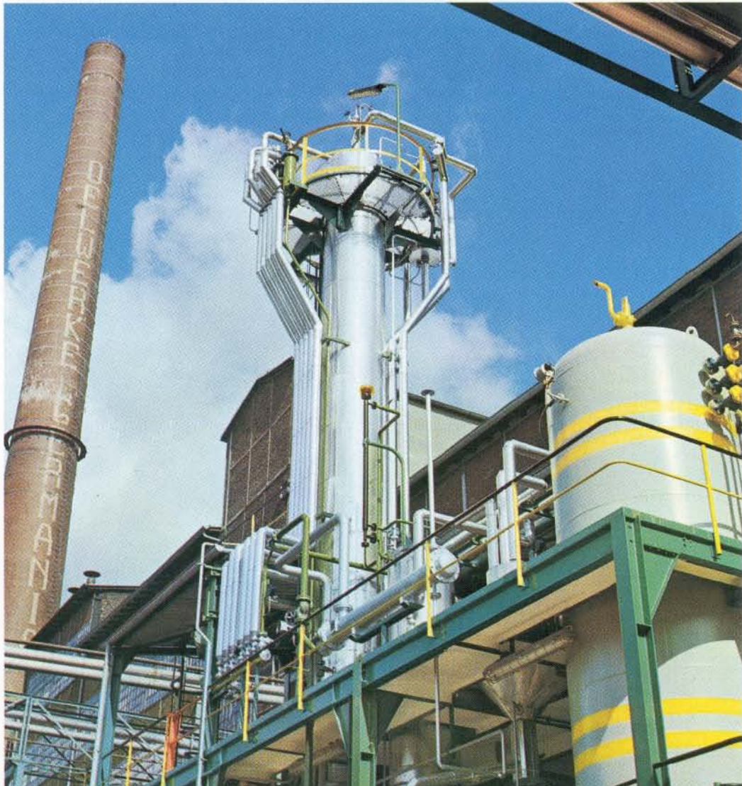
(BELOW) The fully continuous hydrogenation plant, at Oelwerke Germania, Emmerich, Germany.
